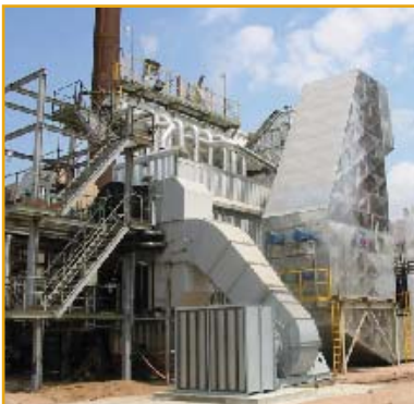
Arab Potash Company, Safi Jordan. Photo from Aalborg Engineering A/S, Denmark.
